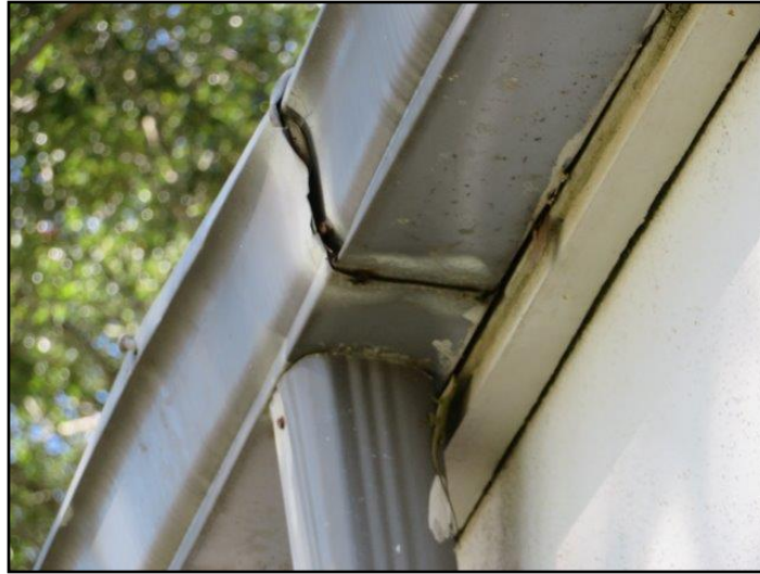
23. Evidence of leakage noted
