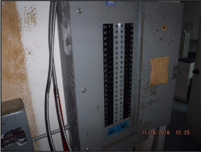
2. Minor deficiencies noted-missing labels
