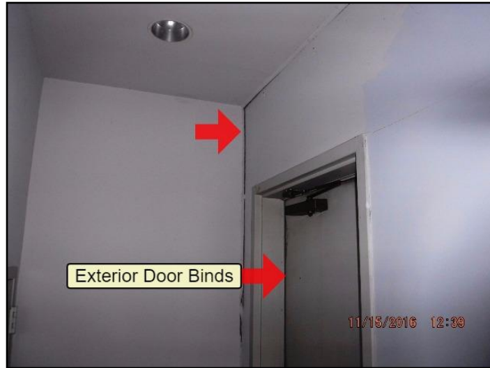
27. Cracked/Separated drywall and doors...
