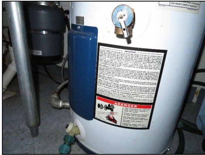
13. Missing discharge from the pressure relief...
