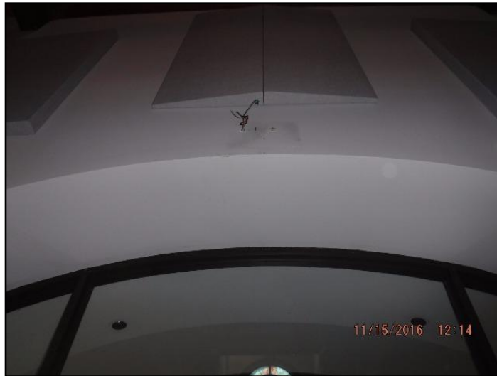
4. Minor deficiencies noted
