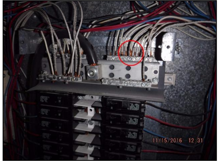
3. Minor deficiencies noted-some wires...
