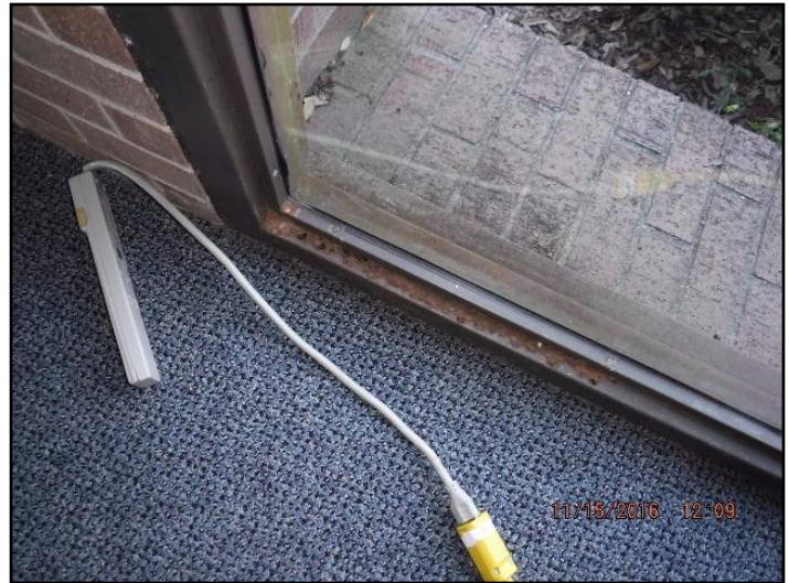
49. Rusted/pitted window frames
