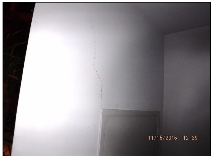
26. Cracked/Separated drywall and doors...
