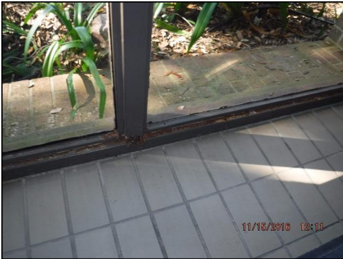
48. Rusted/pitted window frames
