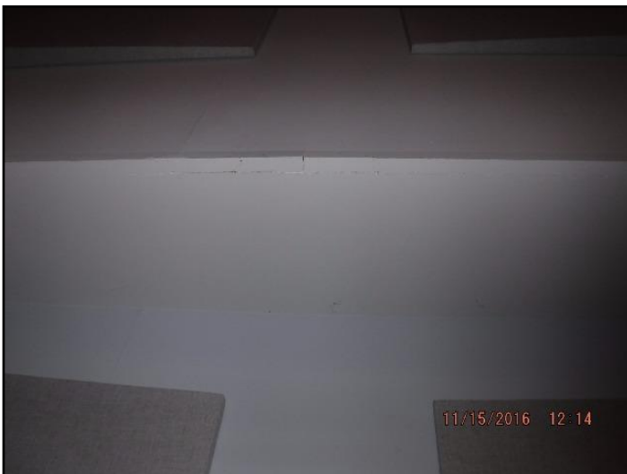
25. Cracked/Separated drywall and doors ....
