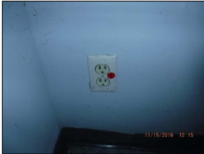
5. Broken blade in outlet near mechanical room
